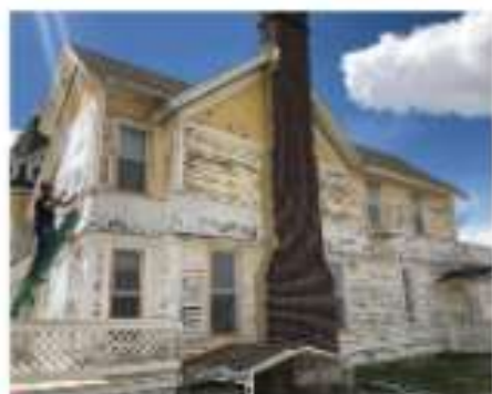
▲ Great plains weather ravaged this 1870s exterior.
